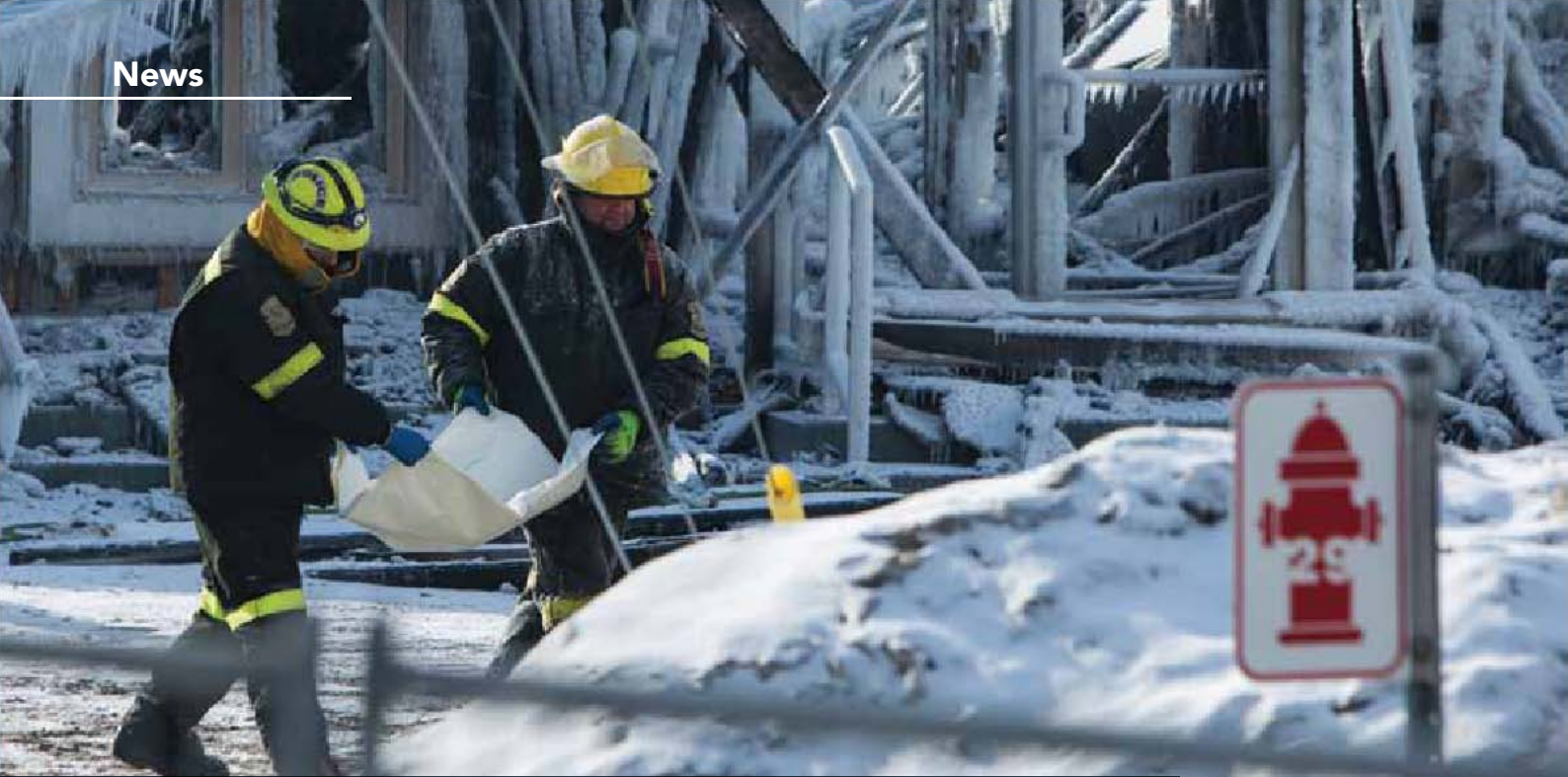
Evidence is pulled from the remains of a fire-charred retirement home in Quebec, Canada
